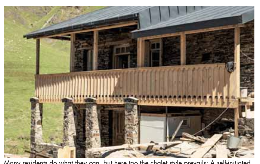
Many residents do what they can, but here too the chalet style prevails: A self-initiated renovation of a residential and stable building from the 1950s in Ushguli
